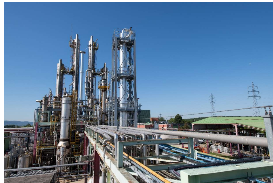
Chemical purification - Speichim (France)
