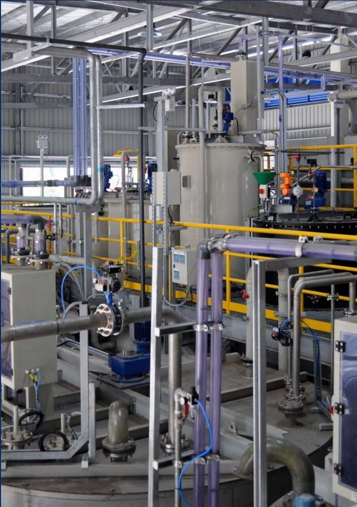
Wastewater sludge treatment - ECO (Singapore)
