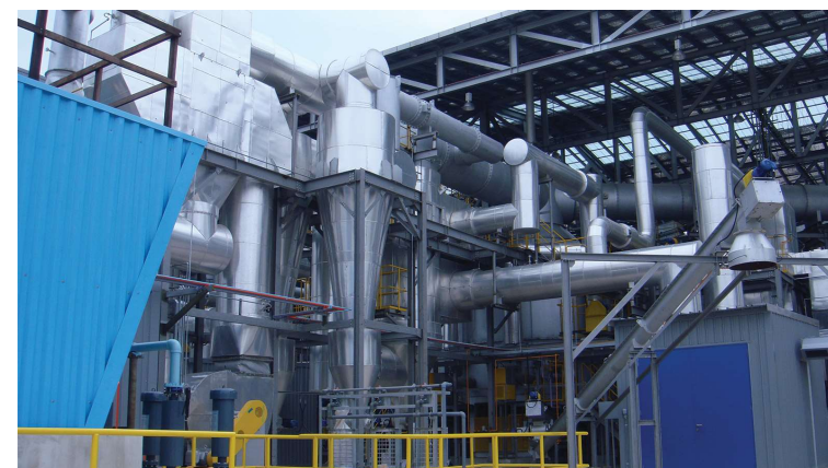
Wastewater sludge treatment - ECO (Singapore)
