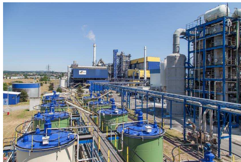
Installations de Salaise-sur-Sanne
